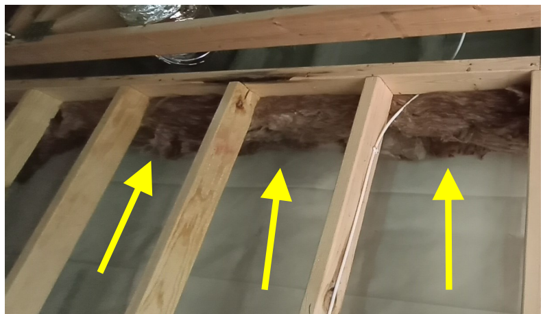
Example of Fire Blocking of furred out wall and ceiling using batts of insulation.
